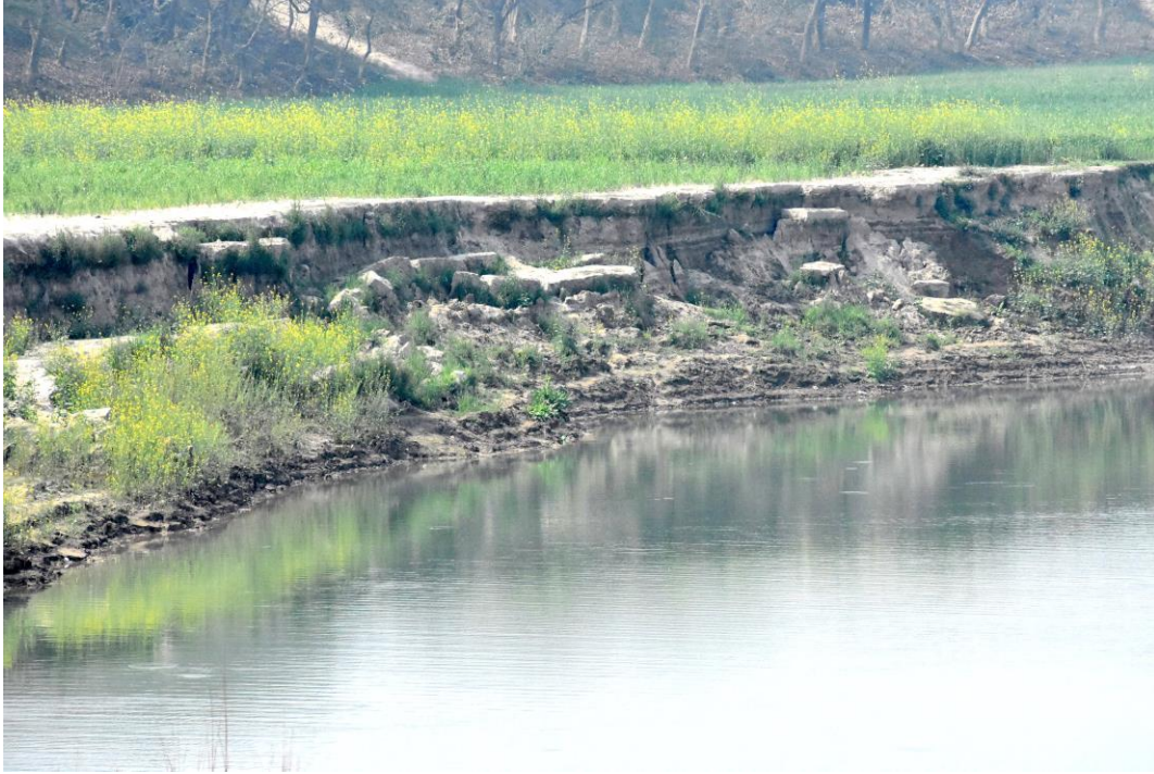
Image 6 : Lateral Bank Erosion Along Ghaghra River As Observed On 16 th February, 2021
