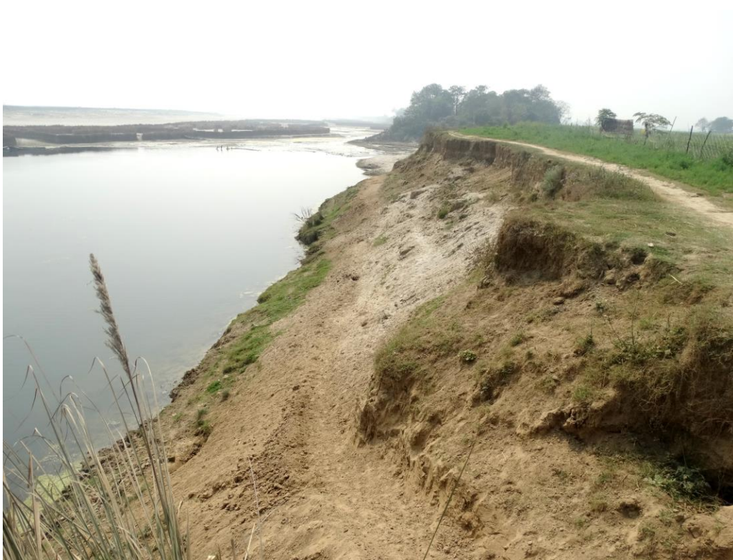
Image 59 : Lateral Bank Erosion As Observed Near Iccha Chaubey Pura
