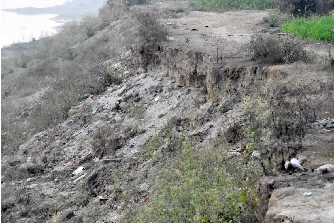
Image 60 : Lateral Bank Erosion As Observed Near Kanspur Ganga Ghat
